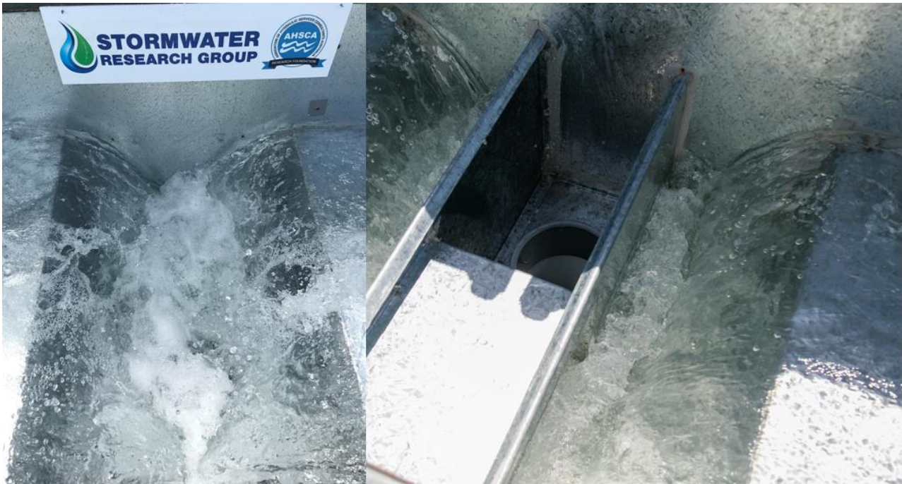
Figure 3 – Highly turbulent hydraulic conditions in sumps receiving box gutter inflows
